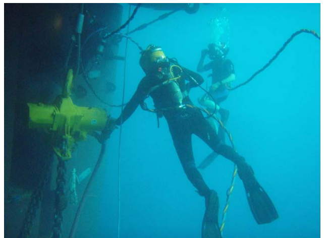
Diver operating a 25 ton air chain hoist during the removal of the rudder
